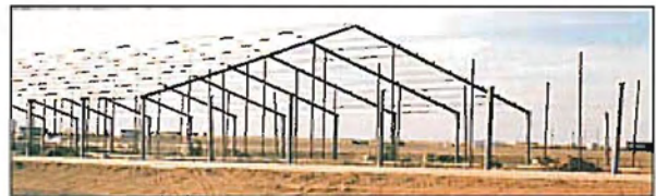
One of Three Freestall Buildings under construction for Mike Schouten, Hereford, TX General Contractor: Mason Dairy Contractors, Amarillo, TX
